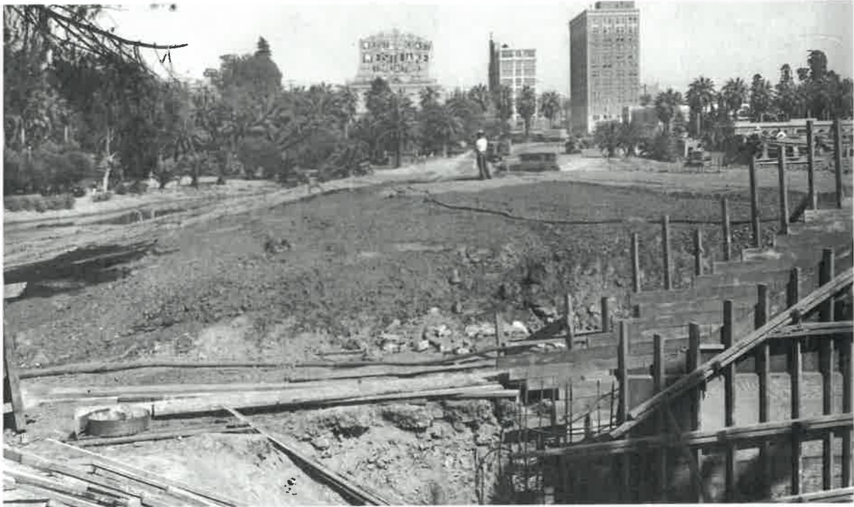
Figure 3. The Construction of Wilshire Blvd. through MacArthur Park looking East, 1934, Photo Courtesy of “Images of MacArthur Park” by Jose A. Gardea, Arcadia Publishing
