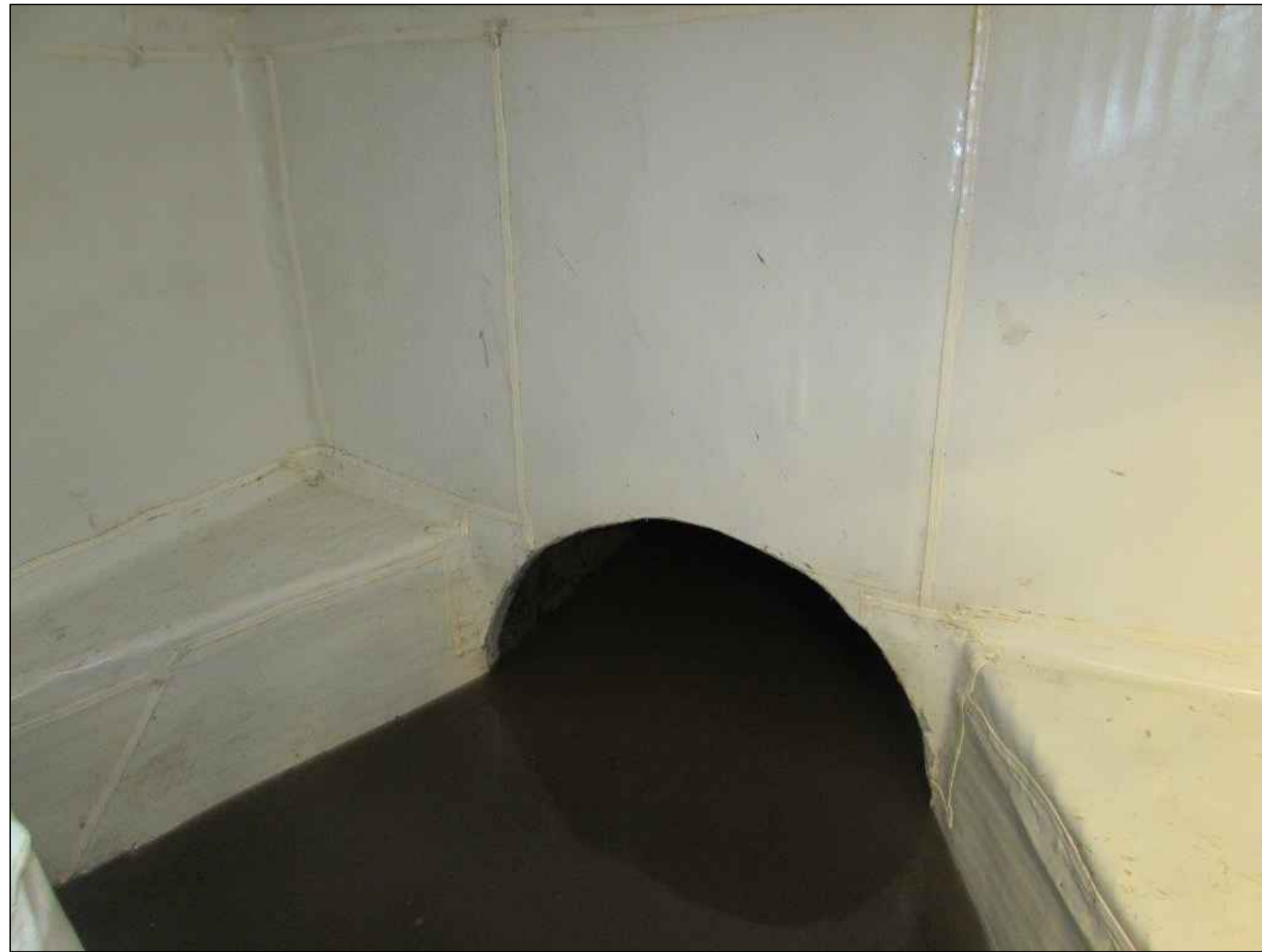
SIPHON INLET (48" SE PIPE)
