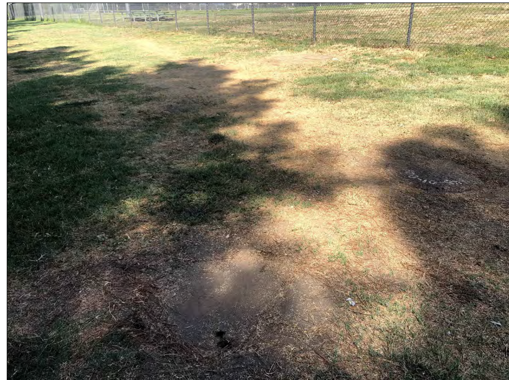
MH #445-01-001 AND TWO ADJACENT MHS
