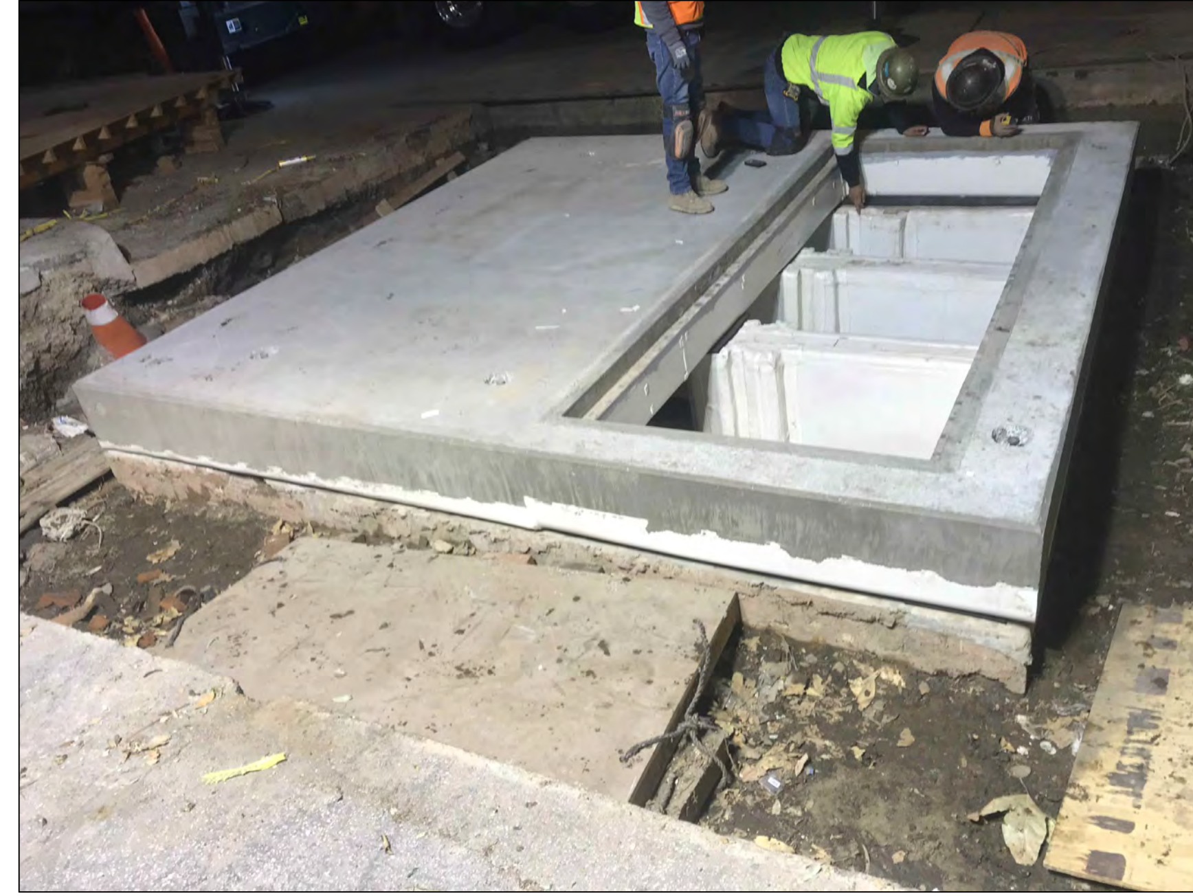
SIPHON OUTLET WITH LID
