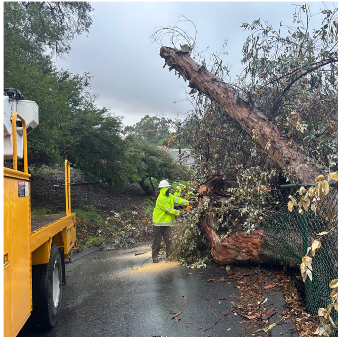
Crews work to clear a downed tree blocking a road.
