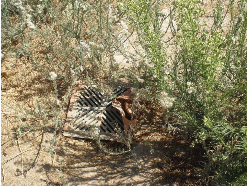
7. View of one of three surface water drains located in middle part of the Site.
