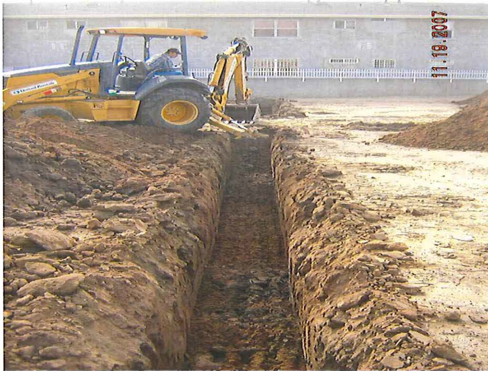
Looking south at a small area of stained soil which was sampled and labeled as S-7
