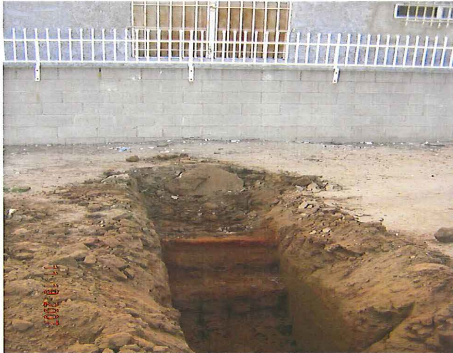
Two abandoned pipelines located on the south end of the property, the upper line is 2" in diameter, and the lower is 3".
