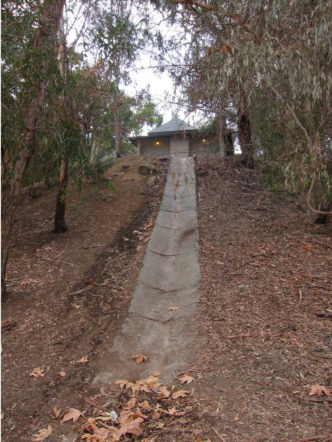
Photo 2: Facing southwest at the drainage located below the restroom building. This drainage appears to be in place to prevent erosion, and to channel water before it sheet flows to the east where it eventually dissipates.
