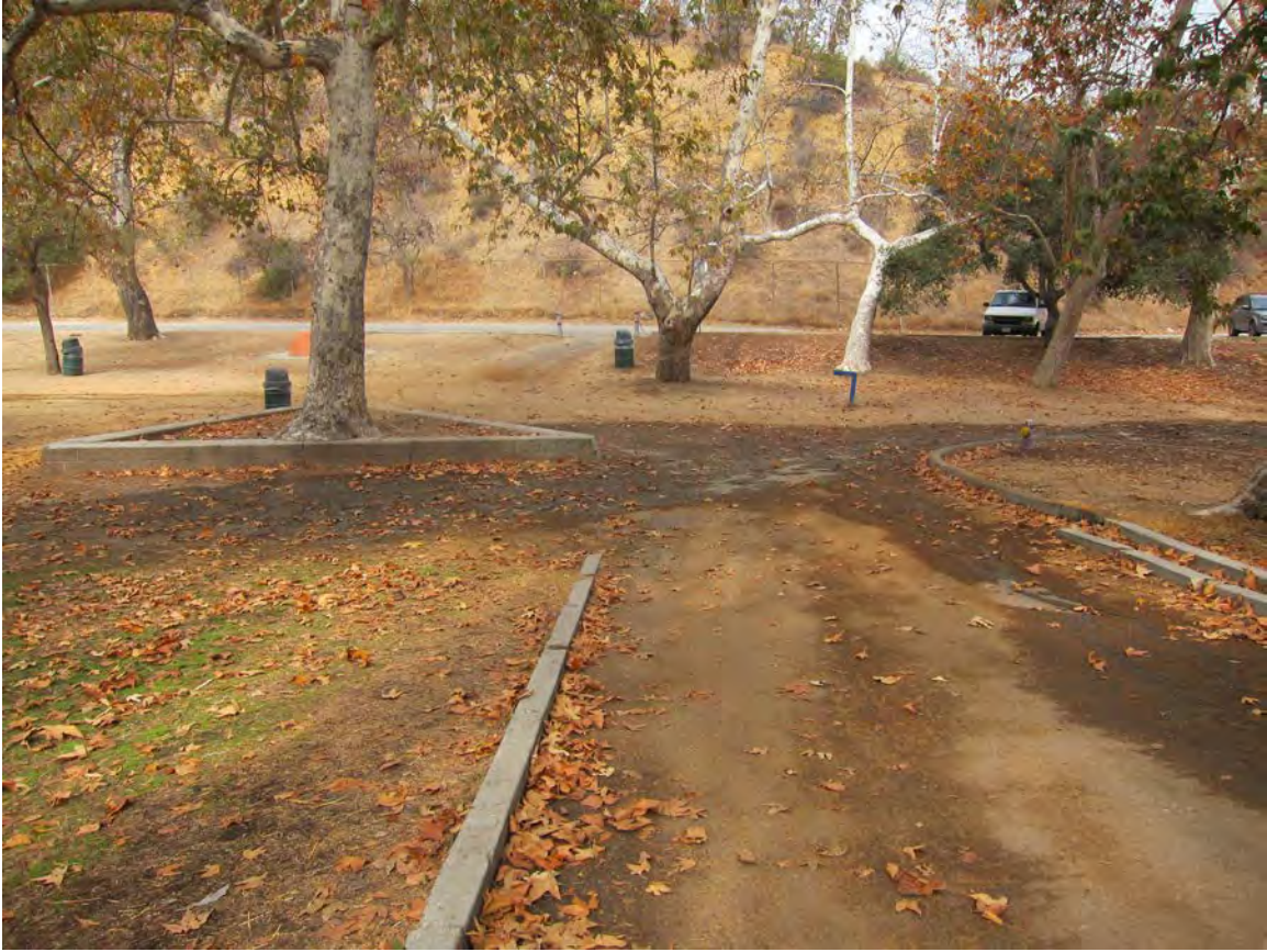
Photo 5: Facing north from the walking path proposed for resurfacing and where the ADA Bridge will be located. This photo depicts a pattern of sheet flows that occurred during a recent rain event.
