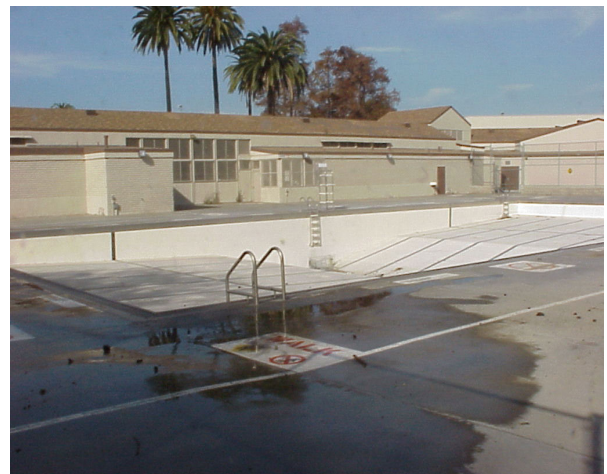
Refurbishment work by Recreation and Parks Facility Repair has kept South Park in good shape.
