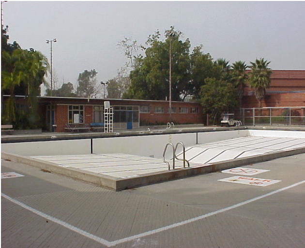
Pool concrete particularly needs replacement at Cheviot Hills.
