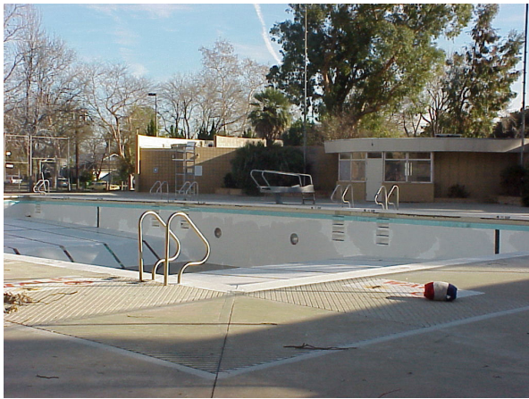
Lanark - Closed, but funding is in place to design and built a replacement
